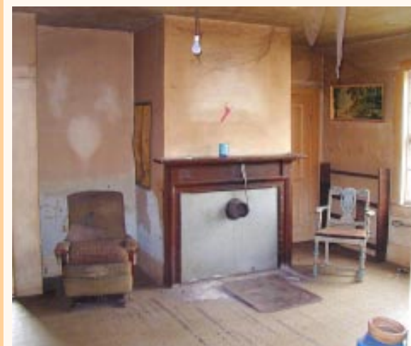
Room 102 – Fireplace hearth footing is river rubble
