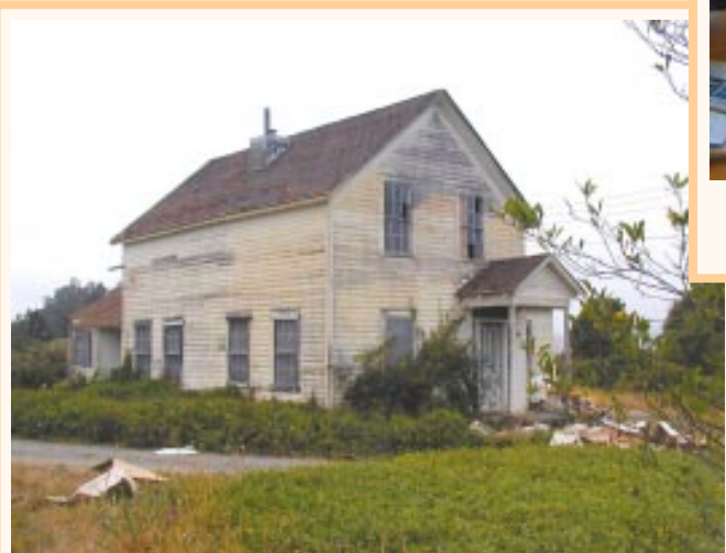
Southeast elevation – Most windows, including entry sidelights need re-glazing.
