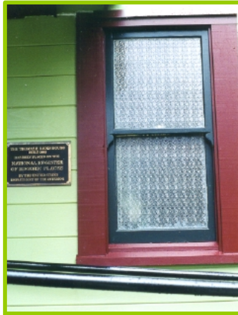
Student built double hung window unit for new ADA restroom (National Register plaque adjacent)
