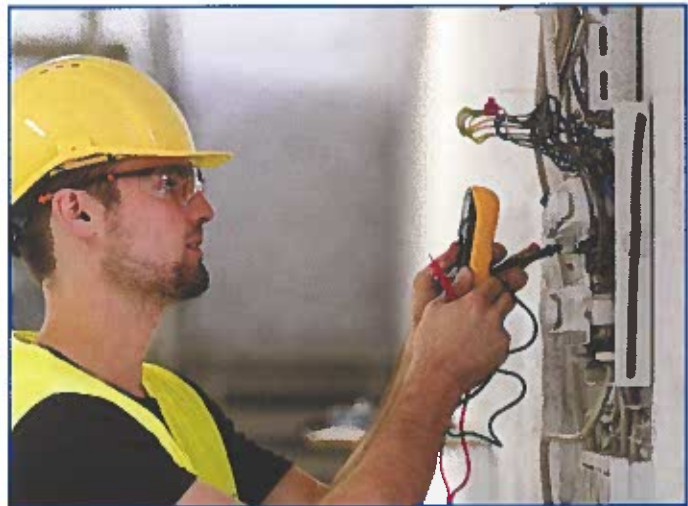
Stay alert for electrical safety hazards
